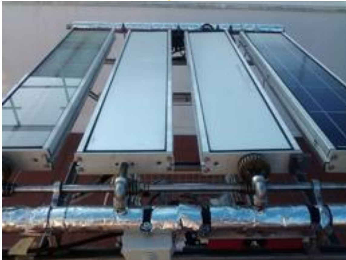
Noon photovoltaic position
